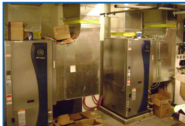
The WaterFurnace Envision heat pumps provide an efficient, reliable and quiet operation for the Mill Bay homeowners.
